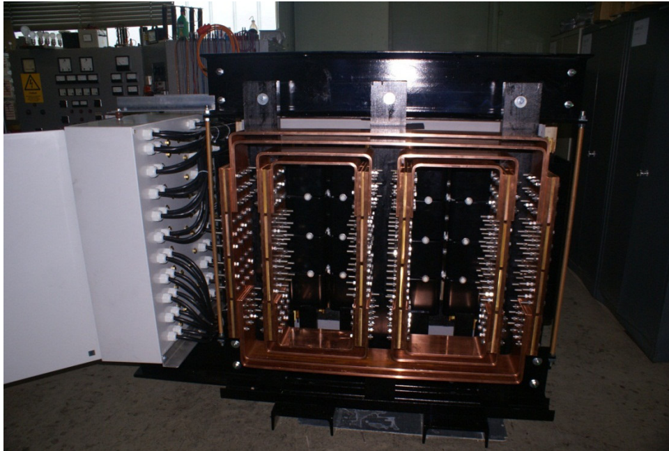
Isolation transformer 800 kVA Primary 3 x 400 Volt; Secondary 3 x .4 .... 19 Volt; 3 x 22790 A Via primary reversible in 10 steps Secondary view
